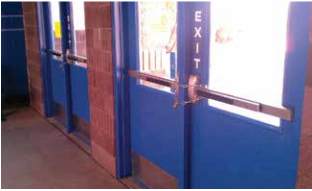
Exit doors in a school, chained to provide security. This locking method does not meet IBC, IFC, or NFPA 101 requirements for egress.
